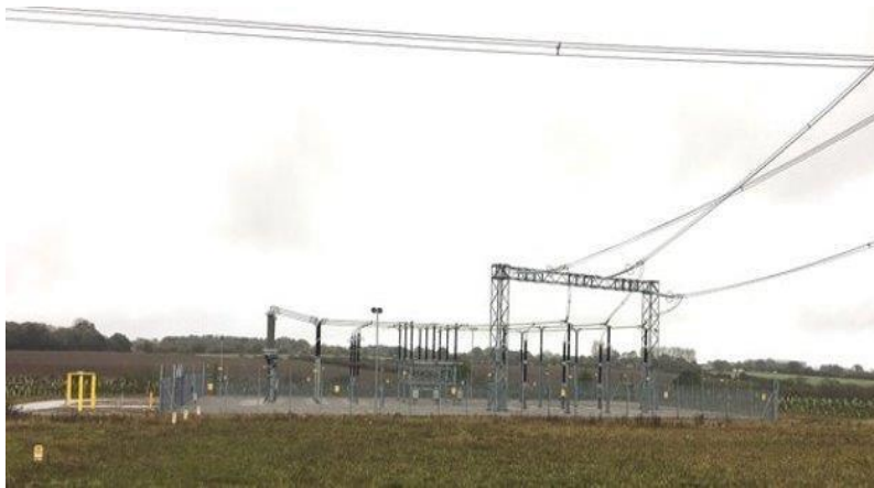
Figure 2.4 Cable Sealing End Compound
